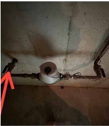
Main water shut-off
