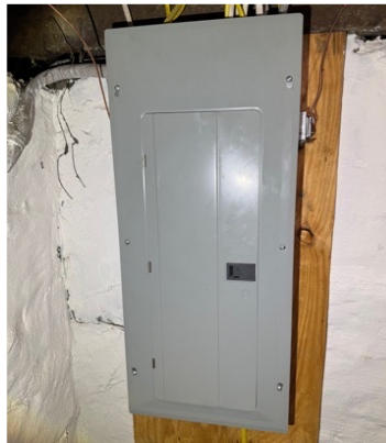
Main electrical panel
