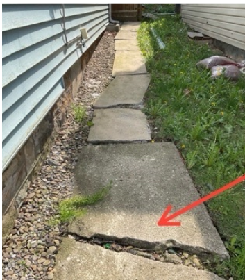
Concrete is cracking
