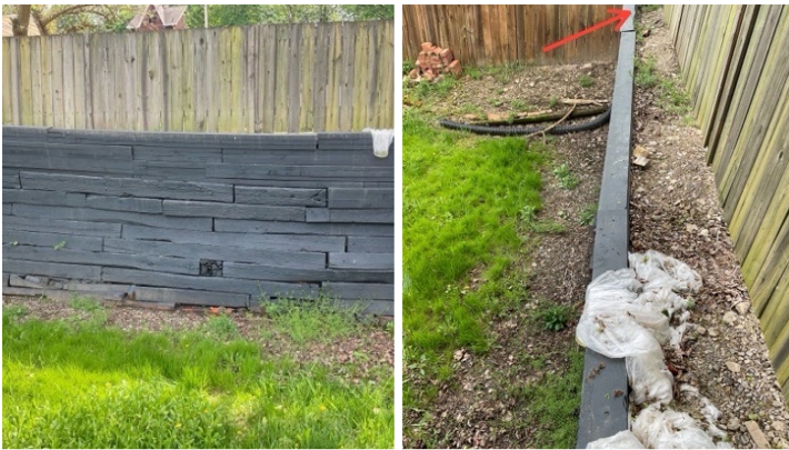
Wall is leaning
