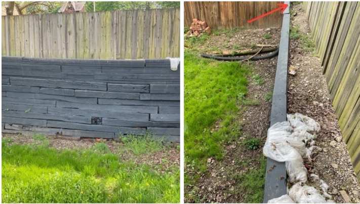
Wall is leaning
