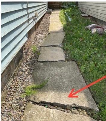
Concrete is cracking
